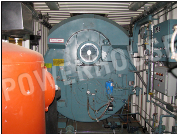
The World's First 800HP Portable Boiler Room
